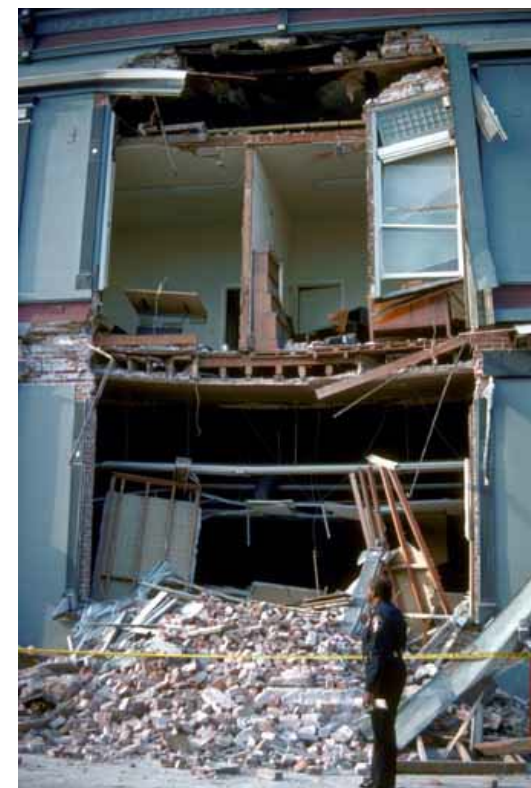
Damaged structure from California's 1989 earthquake
