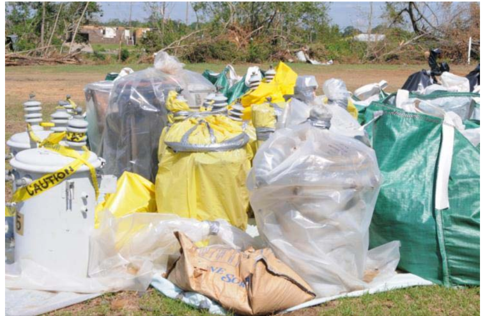
Transformers and other electrical equipment wrapped in bags to prevent oils from leaking
